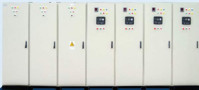
Generator Synchronizing Panel
